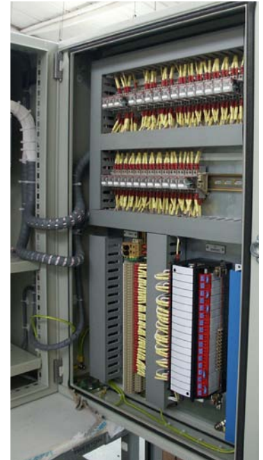
• Conventional Panel Wiring
